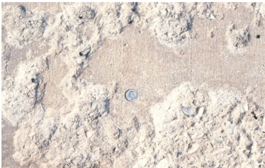
FIGURE 6.4. PORTLAND CEMENT CONCRETE SURFACE SCALING (PHOTO FROM [92])
