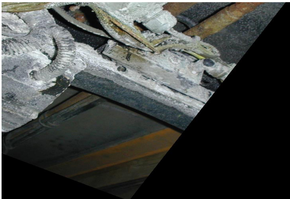
FIGURE 6.14. SALT RESIDUE BUILDUP AND CORROSION (PHOTO FROM [126])
