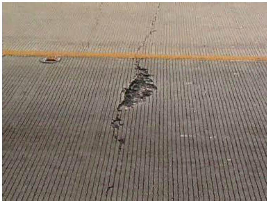
FIGURE 6.8. DELAMINATION AND TRANSVERSE CRACK (PHOTO FROM [93])
