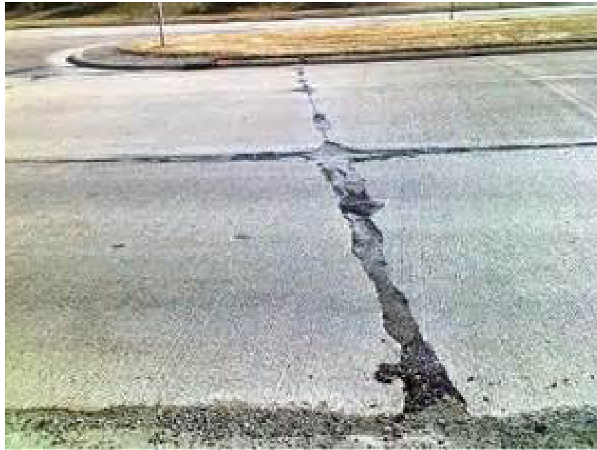
FIGURE 6.7. SPALLING ALONG A LONGITUDINAL JOINT (PHOTO FROM [93])
