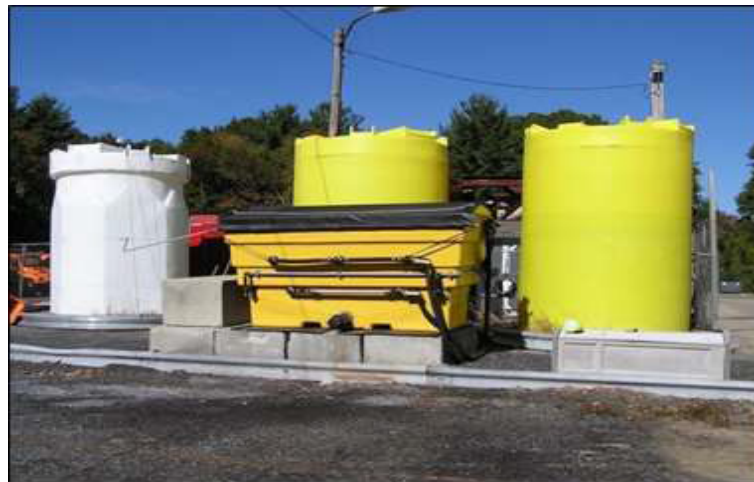
Figure 6: Brine Mixing (Sodium Chloride) and Storage (Sodium Chloride and Magnesium Chloride) Tanks, Putnam Garage
